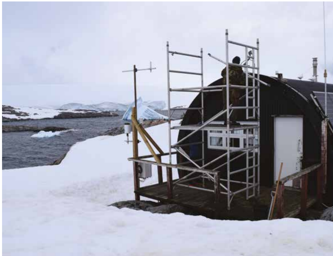
Left New weather station installed
